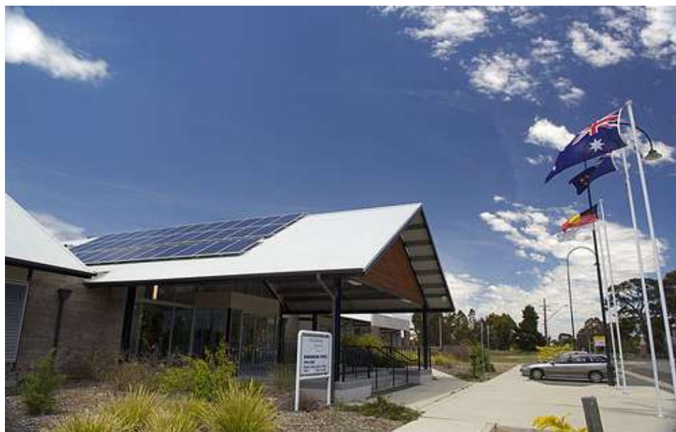
Palerang Council’s recently installed solar PV array
